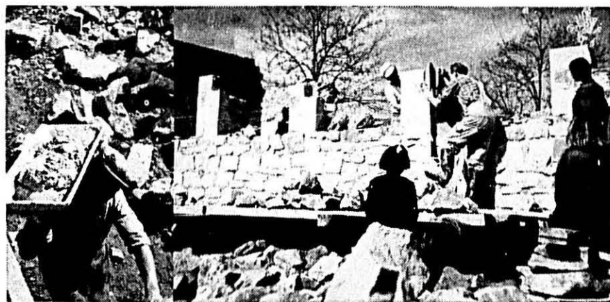
The Greek village of Agnandero had no school. As in many other places its schoolhouse was destroyed during the war. Today, thanks to the contributions of Danish school children and of a team of Danish workers, a new schoolhouse is beginning to rise in the war ravaged Greek town.
